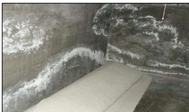
Fig 11.3 Efflorescence in concrete
