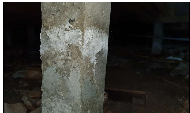
Fig 11.4 Efflorescence in concrete
